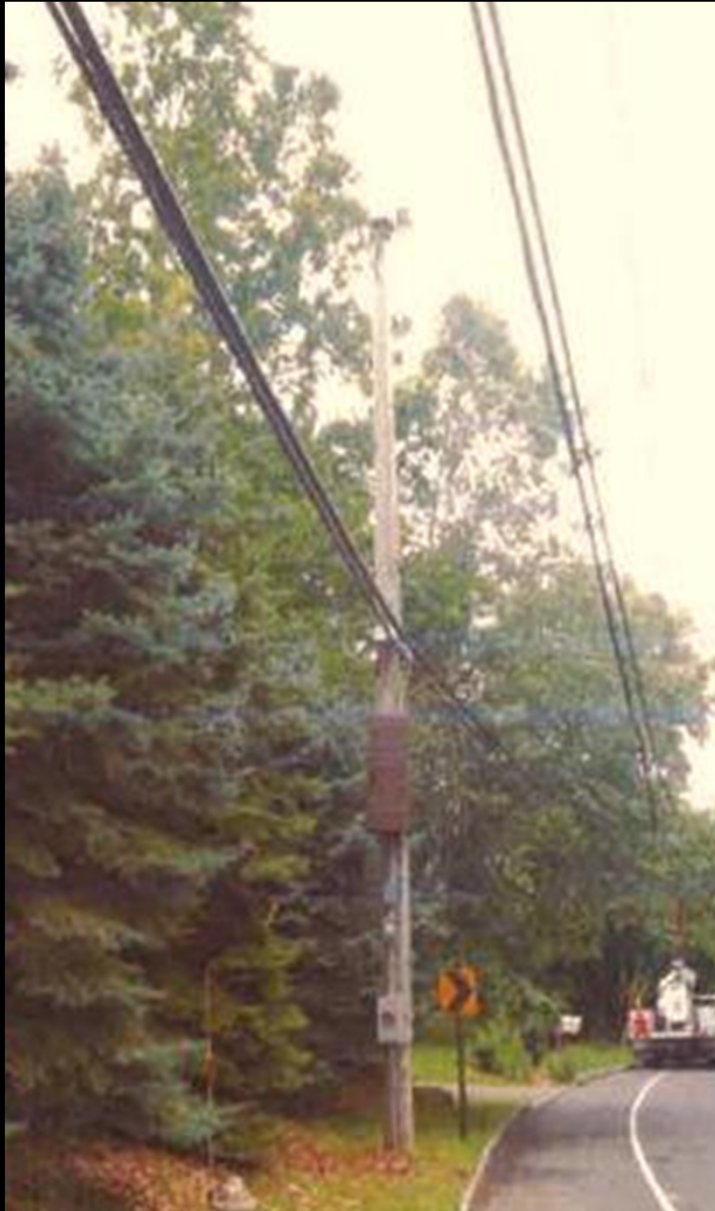
Existing Utility Pole Under 35 ft?
